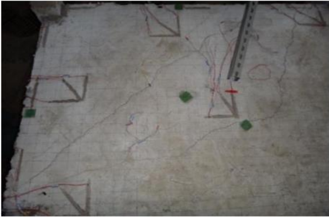
(a) Experimental Cracks of Slab (P1) [20]
