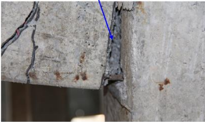
(a) Experimental Cracks at the Longitudinal Beam [21]
